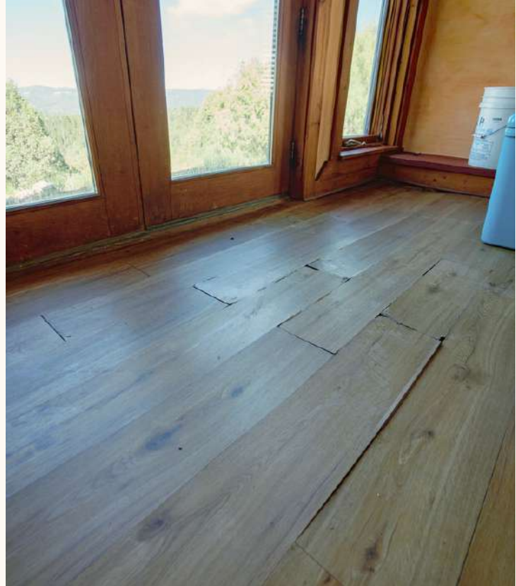
Floor showing the wear of time, awaiting renewal
